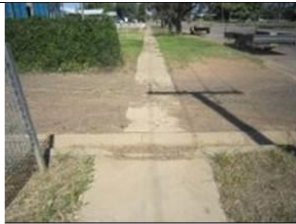
4. Loose gravel from a mid-block laneway creates a trip hazard for all pedestrians.
