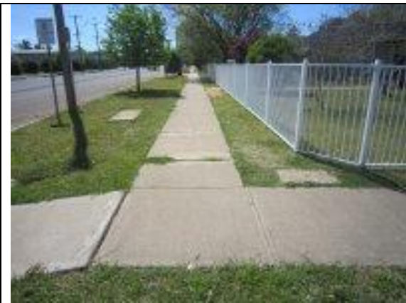
7. Grass in footway joint.
