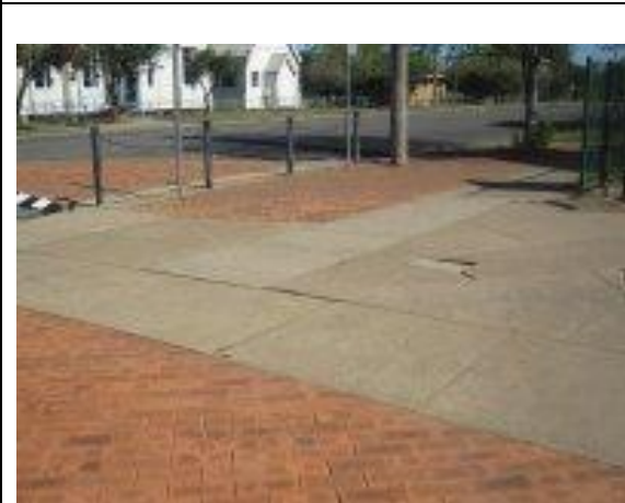
9. Telstra pit dropped at entrance to Church.
