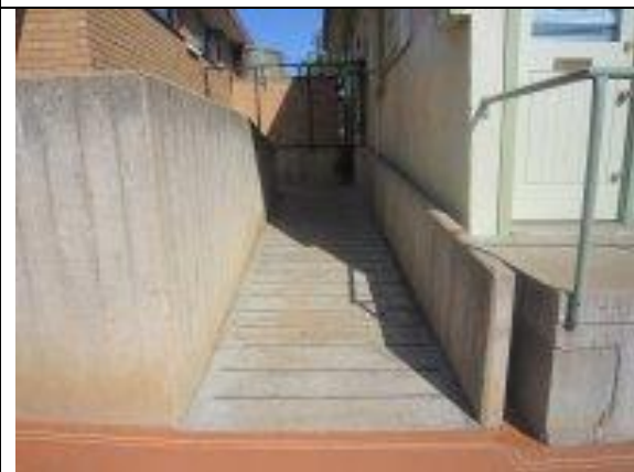
19. Handrails are required on both sides of a ramp.
