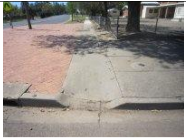
12. Narrow kerb ramp with steep splay.
