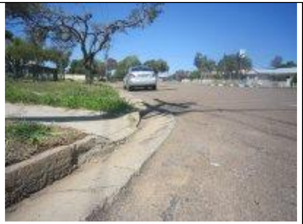
14. Kerb ramp and gutter are both very steep, creating a tip hazard for wheelchairs.
