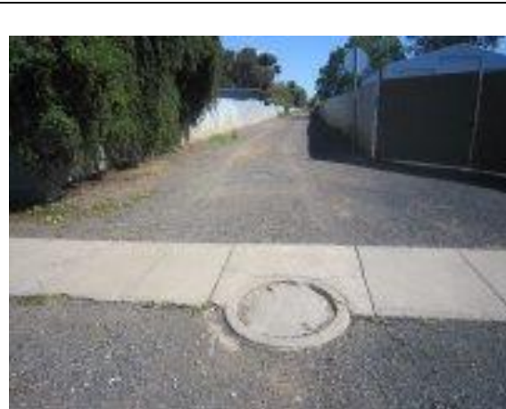
10. Manhole collar and lid damaged.
