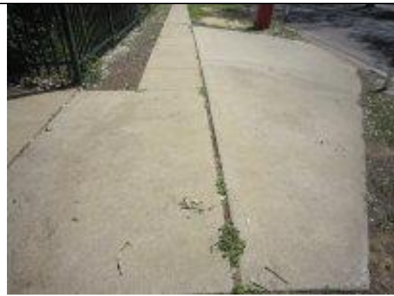
8. Wide joint in footway.
