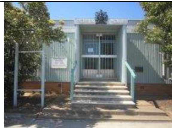
17. Steps are required to have handrails on each side.
